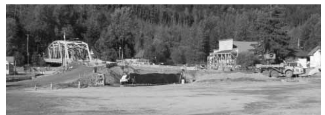
Backfilling and restoration work near the intersection of 5th Street and Railroad Avenue in mid-September.
