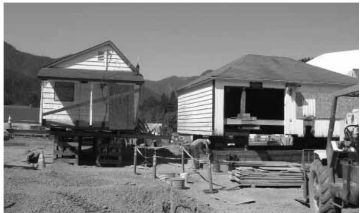
In August, crews started work on foundations for homes on 4th Street.
