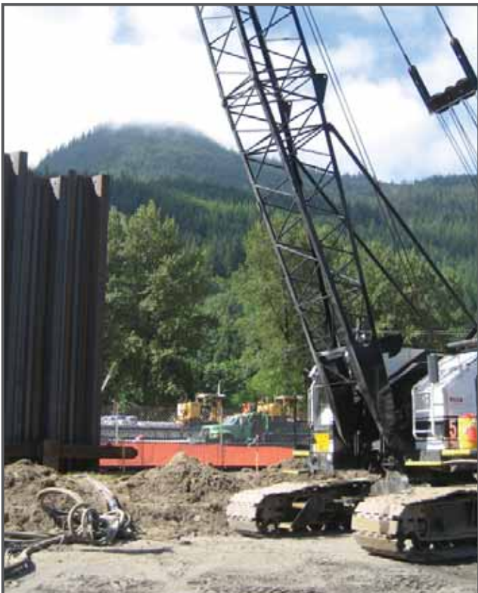
View of sheet pile installation at the east end of the construction area.
