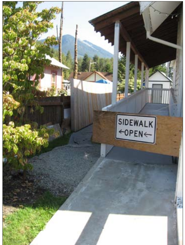
The temporary pedestrian walkway was installed near the Skykomish Church during early September.
