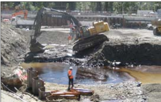
Crews recover oil from Railroad Avenue and 4th Street.
